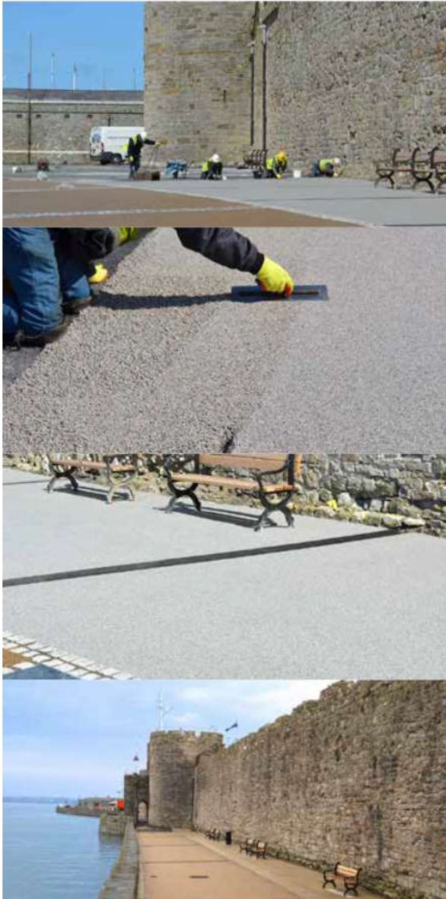
Meon DekorGrip Resin Bound Surfacing at Caernarfon Castle, Wales – Grey and buff colour schemes
