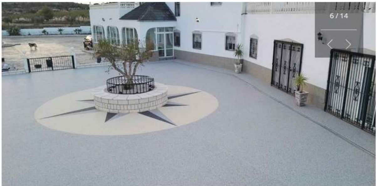
Addagrip Addabound Resin Bound Surfacing with recycled aggregates – Grey colour with light buff colour and decorative shapes
