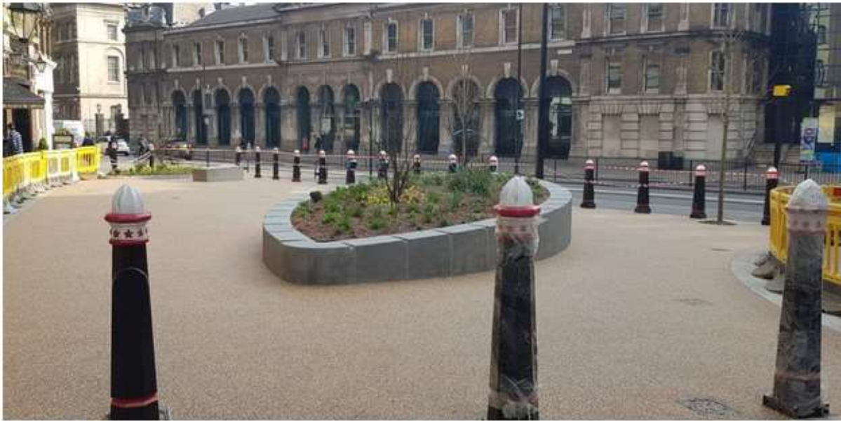
Addagrip Terrabound Resin Bound Surfacing at Monument Street, London – Peanut colour scheme
